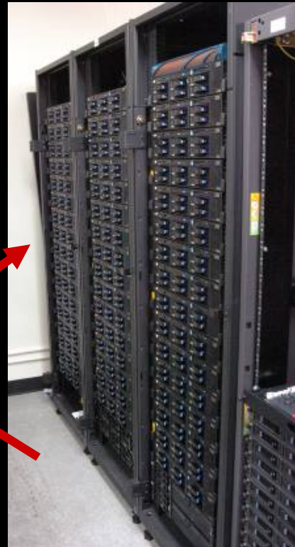
IBM Storage Cluster
